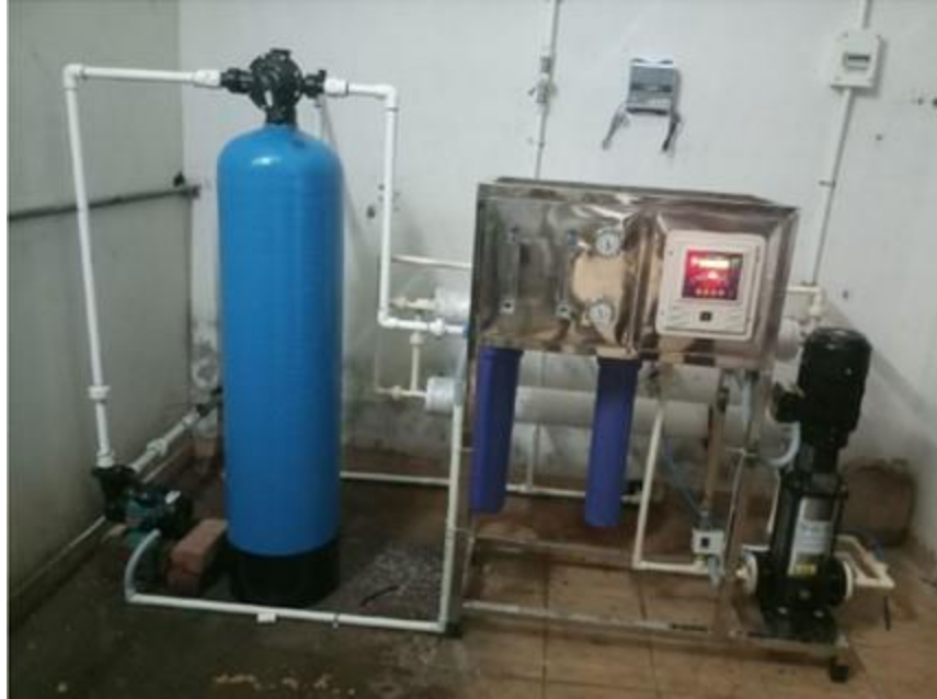
RO Water Plant for clean drinking water
